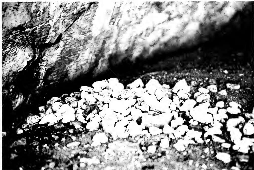
Photo 26. View showing crushed rock forced out of weep hole. Bledsoe Street undercrossing of Foothill Freeway [36].
